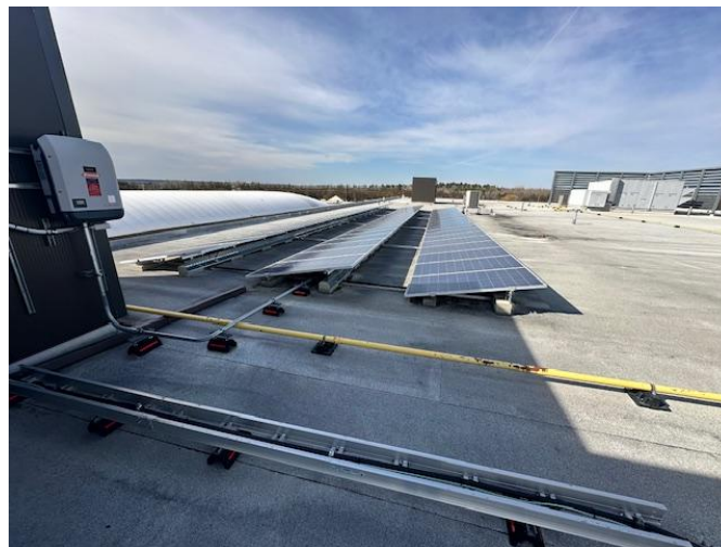
Picture 12. Skills Building Solar Panels
